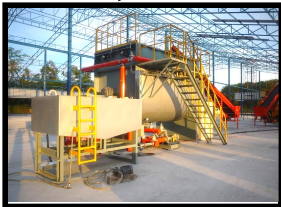
The digester, which works at 80°C to break down organic waste into fertilizer, is an integral part of Biomax process
